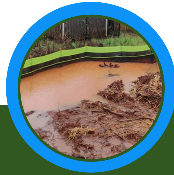
Two-stage Flow Silt Fence
